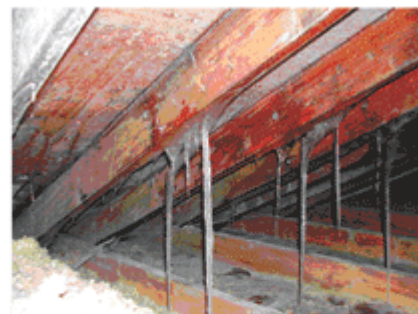
Condensation resulting from excess moisture being dumped into the attic has frozen on the underside of the roof sheathing.
