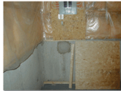
Notice the patched hole in the foundation below the electrical panel where stolen power was brought into the home.
